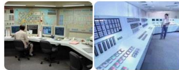
(DCS central chiller plant control room)
