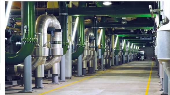
Chiller room inside the largest district cooling plan in the world, at The Pearl-Qatar. (Image courtesy Qatar Cool)
