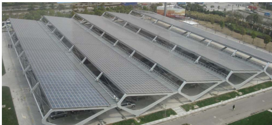
Fig. 48 Photovoltaic Carports with Double-Glazing Module
