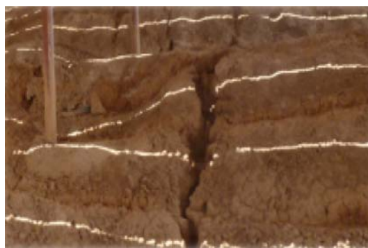
Figure 4-26 Inadequate Preliminary Preparation
