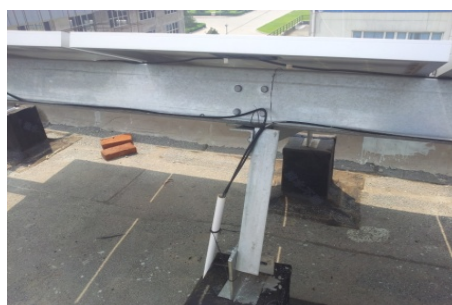
Figure 4-33 Inappropriate Cable Protection
