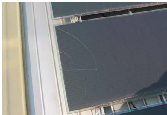
Figure 4-12 Glass Panel Fracture
