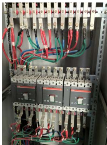
Figure 4-23 Failure to Install Breaker Phase Partition
