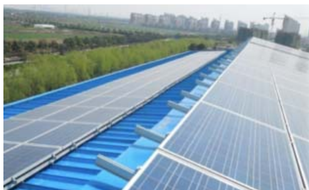
Figure 4-24 Unreasonable Dip Angle Design
