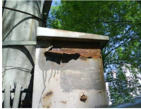
Figure 4-20 Protective Shell Coating Quality Problem
