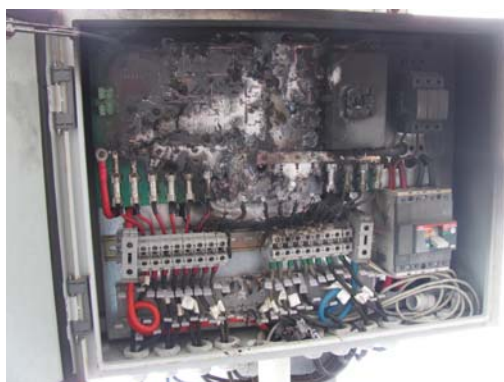
Figure 4-16 Burnout Caused by Insufficient High Voltage Creep Age Distance
