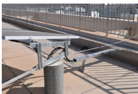
Figure 4-34 No Cable Protection
