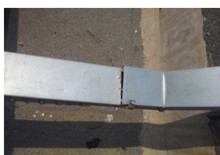
Figure 4-35 Trunking opening quality
