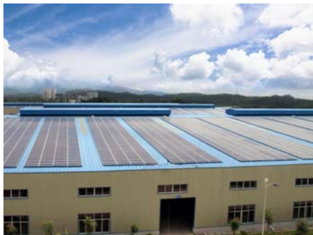
Figure 2-6 Self-provided Commercial and Industrial Power Plant (Distributed)
