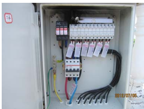
Figure 4-17 Short Circuit Burnout Due to Unreasonable Structural Layout
