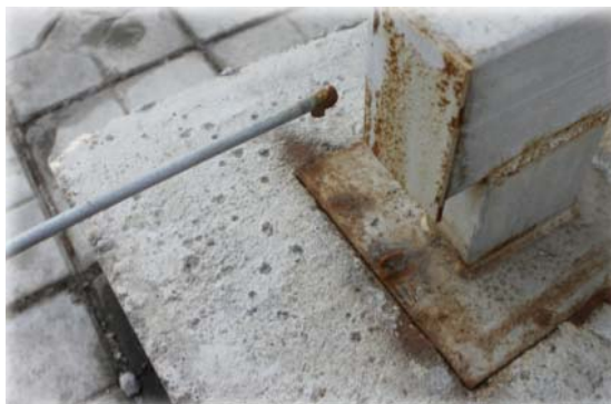
Figure 4-28 Unreliable Equipotential Connection Welding
