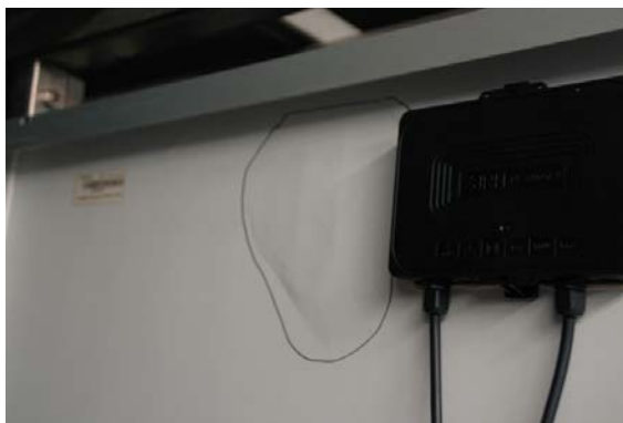
Figure 4-10 PV Module Rear Panel Bump
