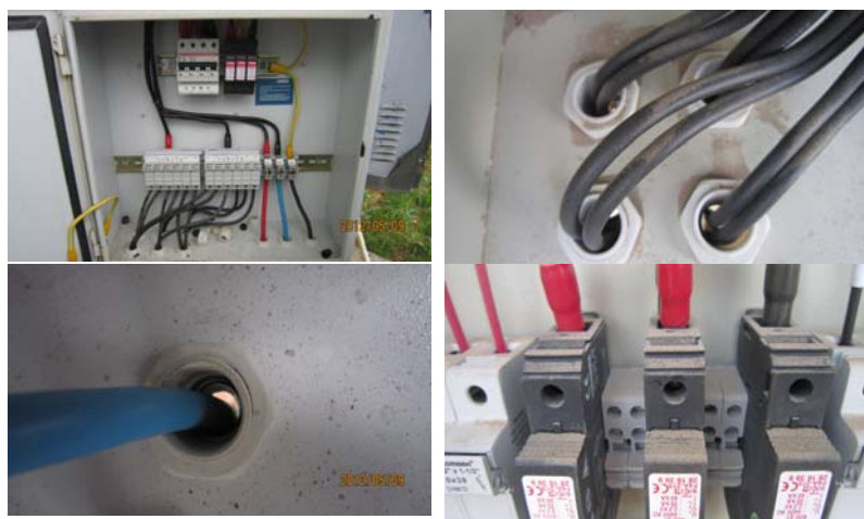
Figure 4-22 Nonconforming Inlet Wire Installation
