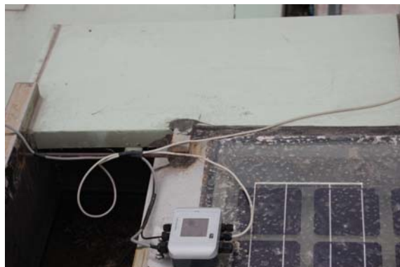
Figure 4-40 Early Burn-in of Irradiator Wiring
