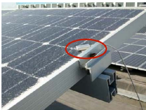
Figure 4-44 Failure of Sticking the Temperature Sensor to the Rear Panel
