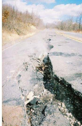
Figure 4.25 Subsidence above an underground fire in Pennsylvania (USA), (ISRM, 2008)
