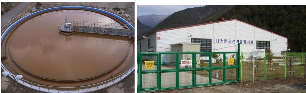
Figure 4.15 An active treatment facility of the abandoned coalmine in Hamtae (left) and electro dialysis treatment system in Najun coal mine
