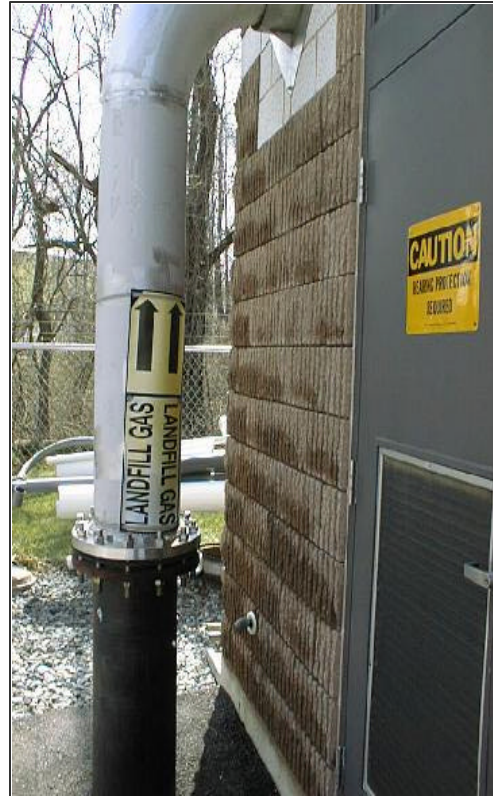
Figure 18: Landfill Gas Intake Pipe
