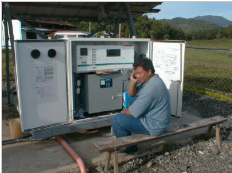
Figure 14: Technical Manager with Power System and Cell-phone
