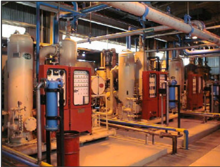
Figure 19: Landfill Gas Processing Facility
