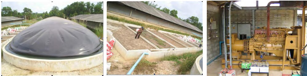
Fig 10. Channel Digester System in Case Study Site
