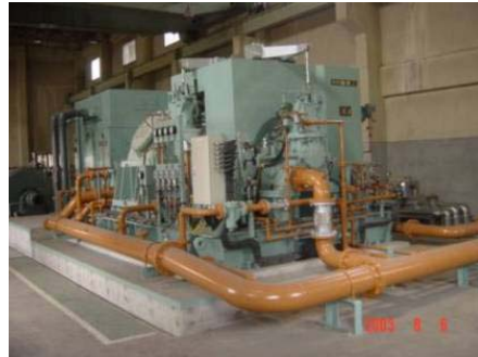
No.2 Steam Turbine (10,200kW)
